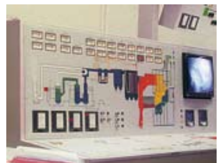
Figure 3: Control Room Featuring M1000 Process Alarm Monitors.
